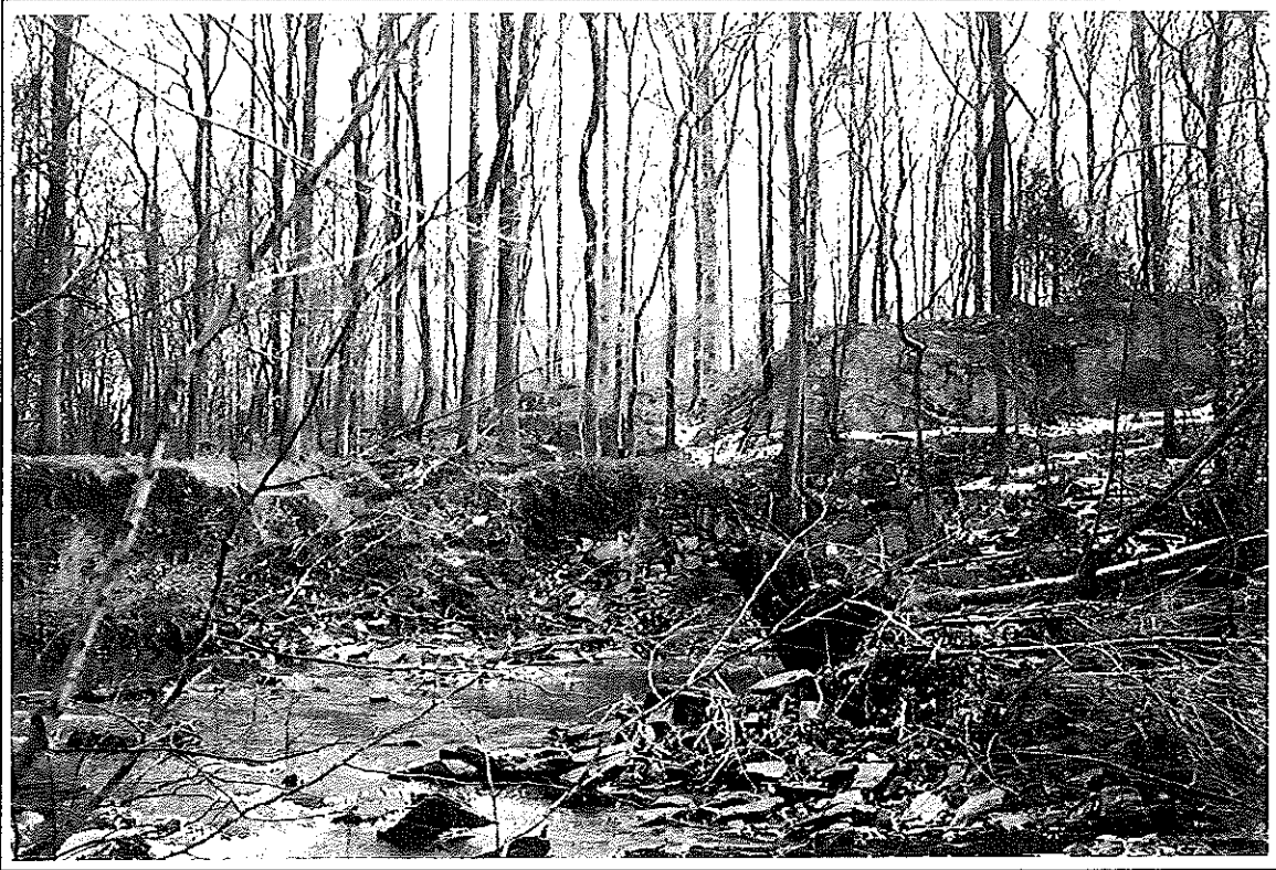
Cook's Mill (#E). Broken dam across Mill Creek.
